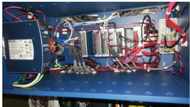
FIG. 4. Inside of installed Hardware Interlock System crate.
